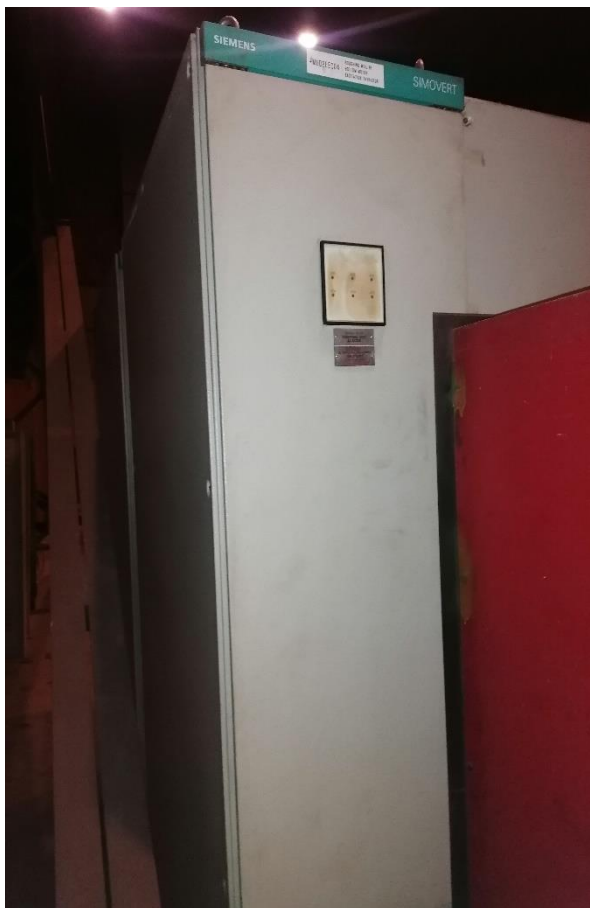
Slika 2 – Cabinet for field regulator for TOP motor
