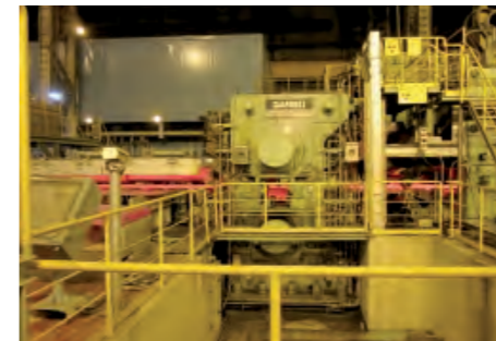
Crank shear in operation (Far East).
